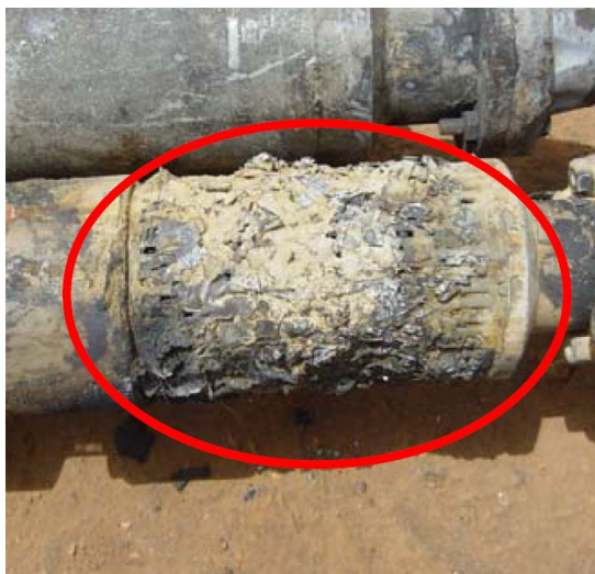
Figure 3. Calcium carbonate \text{CaCO}_3 scale blocking pump intake [14].
