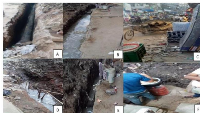
Fig. 2. Pictures from pipeline repair pit from which the soil tested positive for the soil-borne pathogen B. pseudomallei
