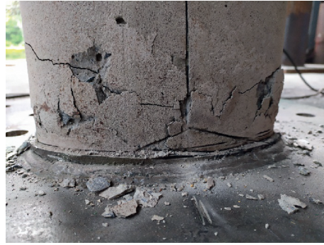
FIGURE 8: Typical damage mode of the concrete.
