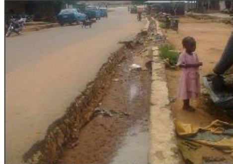
Plate 2 Showing the presence of edge crack defect with high frequency thereby leading to the collapse of the drain wall. (Kelebe Road).
