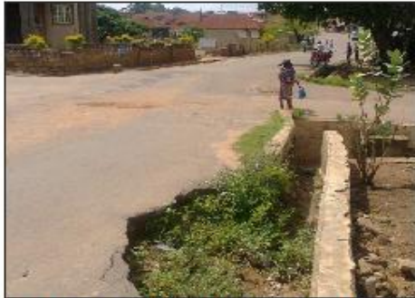
Plate 1 Showing the presence of edge crack with high severity (Kelebe Road)
