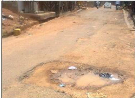
Plate 4 Showing pothole with medium severity (Olode road)
