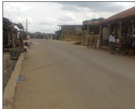
Plate 6 Showing a good section of a pavement with adequate drainage facility (Jamodo - Central Mosque road).
