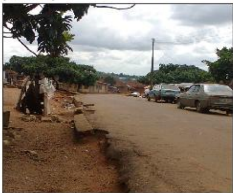
Plate 5 Showing the presence of edge crack defect and the absence of line drain (Elder Akande road).
